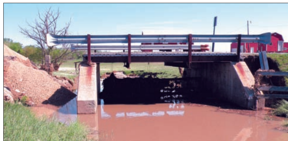
County engineer Paul Coutts described the damage to CR200 (the Crooked Road to Flora/Delphi) at the commissioner's meeting Monday, but words cannot do justice to the devastation done to the road during the Friday night deluge. Storms traveled through the county dropping, in some places, more than 5 inches of new water on already saturated ground. The water found its way through the ground, washing away soil and undercutting the road that left the asphalt with no support. Photo provided
