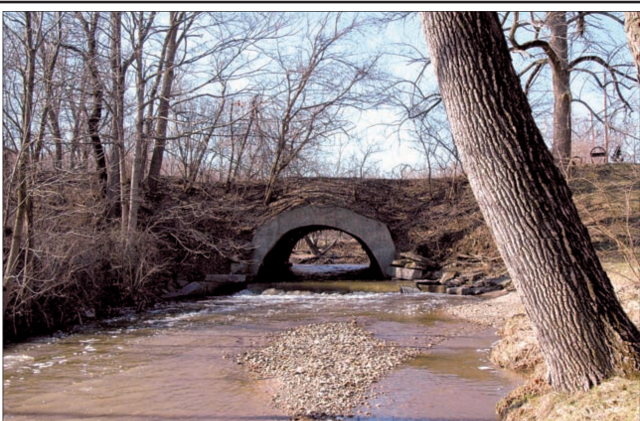
A glimpse of history Burnett's Creek Arch, the oldest stone arch bridge in Indiana, is located on Towpath Road in Adams Township. It appears on the National Historic Register as the "Wabash and Erie Canal Culvert #100." Comet photo by Debbie Lowe
