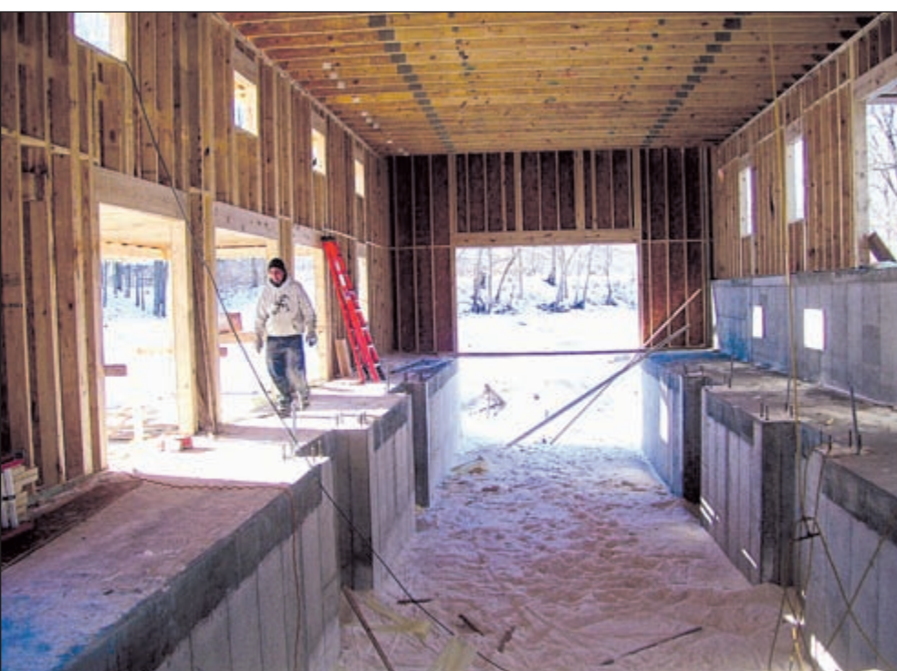
This "slip" (dry today because the canal was drained) inside the warehouse will safely store the new boat. It will allow raising the boat above the water level in winter to protect the hull from ice damage. Photo provided
