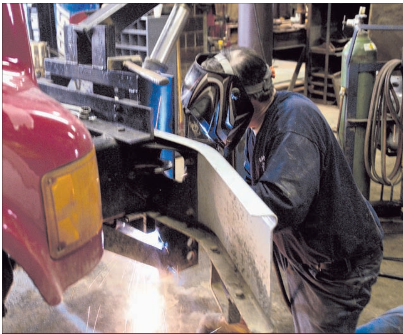
Tom Shockley, Carroll County Highway Dept. employee, repairs a snowplow carrier by welding on a new brace cut from square tubing. He said the cold weather is hard on equipment. More snow flurries and frigid temperatures are expected this week. Comet photo
