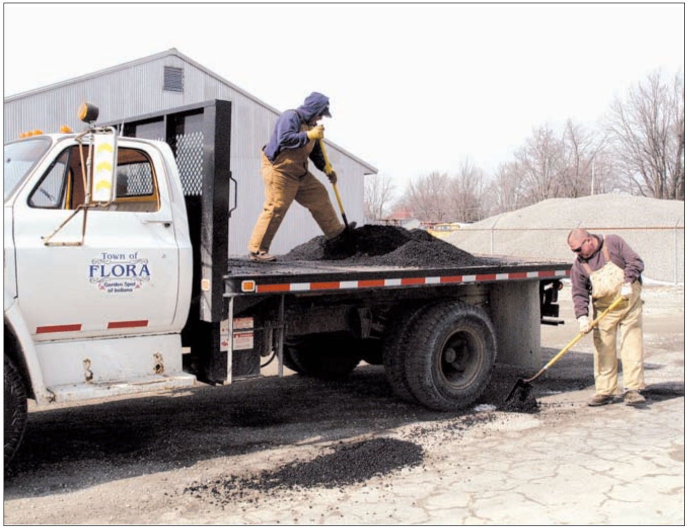
Flora town employees Darrell Hoffman, left, and Greg Barnes, right, worked Tuesday repairing potholes on town streets with cold patch. They were making repairs on South Third Street in front of the County Highway Garage when this photo was taken. County workers are also out repairing roads this week. Comet photo
