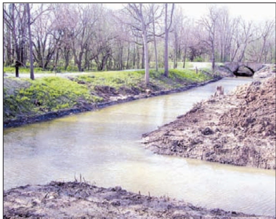
Canal work A visible difference can be seen in the canal waterway off Bicycle Bridge Road in Delphi. Workers have removed tree remnants and debris, and restored the canal to look more like it once did. Work is also being done on the canal sidecut, pictured lower right, which once took boats to the foot of Main Street. In a couple of years, the Wabash & Erie Canal Association expects to have its own replica canal boat. Photo provided
