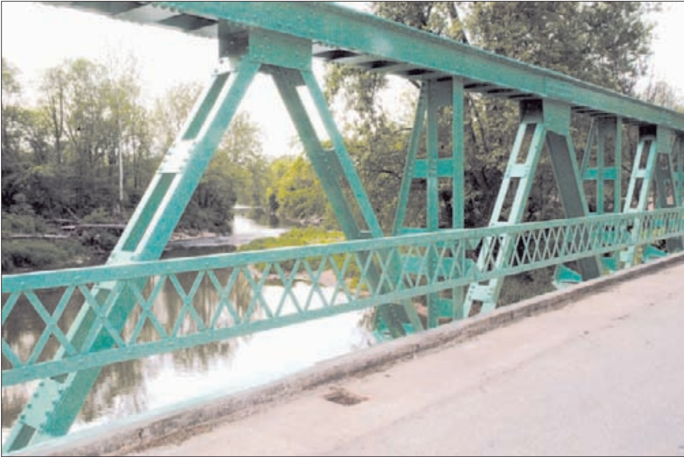
The structure long known as "the green bridge" on Meridian Line Road near SR 218 now lives up to its name. Before being recently painted, the pony truss bridge was mostly rust-color. Carroll County Highway Supt. Ron Francis said the new coat of paint and some structural repair work came about as part of the overall bridge maintenance schedule. A painting contractor put a tent over the bridge before sandblasting in order to meet environmental guidelines for reclaiming the old paint. Comet photo by Jennifer Archibald
