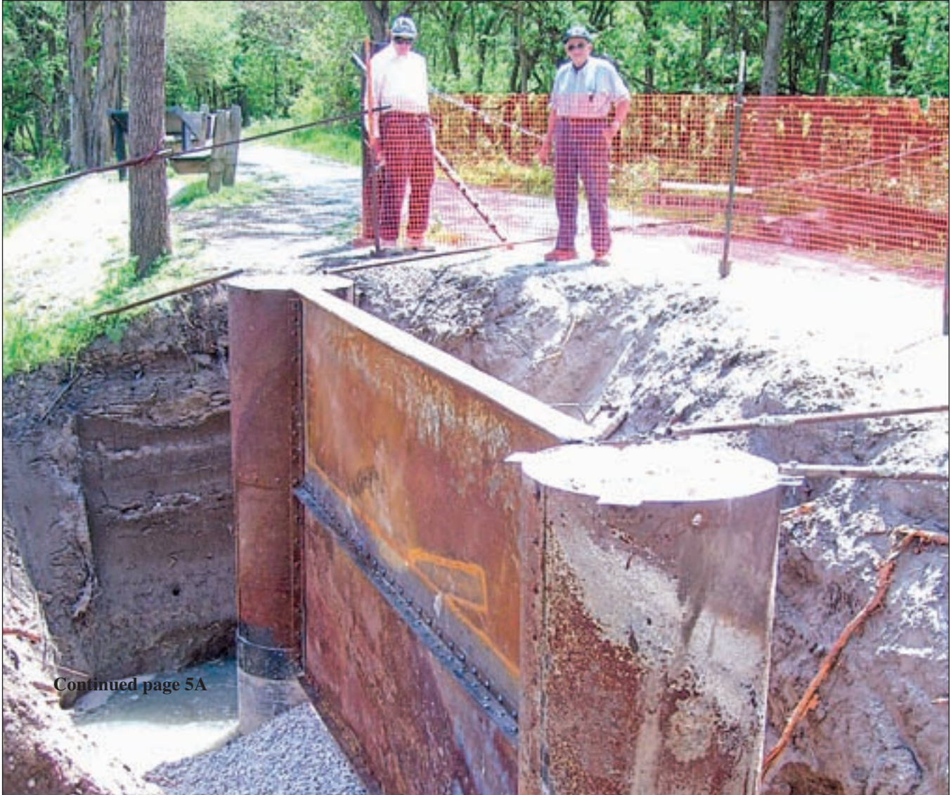
Canal volunteers have been busy restoring the 1905 Stearns iron bridge obtained from Pulaski County last year. When assembled, the bridge will span the canal behind Dairy Queen in Delphi. This photo shows one end of the bridge foundation that was recently installed deep into the west side bank. The location is off Bicycle Bridge Road, along the Vanscoy Trail. Pictured l-r are Ron Dust and Bill Draper. Recent work on the bridge has included cleaning and painting the 100-plus pieces of wrought iron making up the 78-foot long structure. Photo provided
