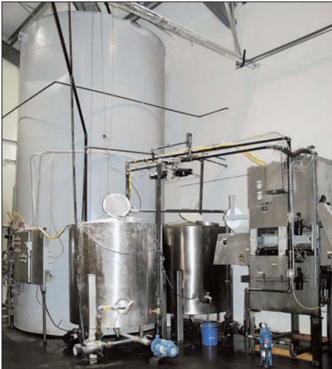
B100 storage tank
